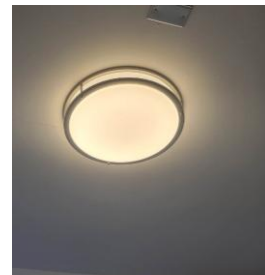
New Light Fixtures
