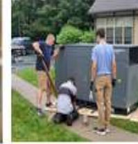
Our New Generator is installed
