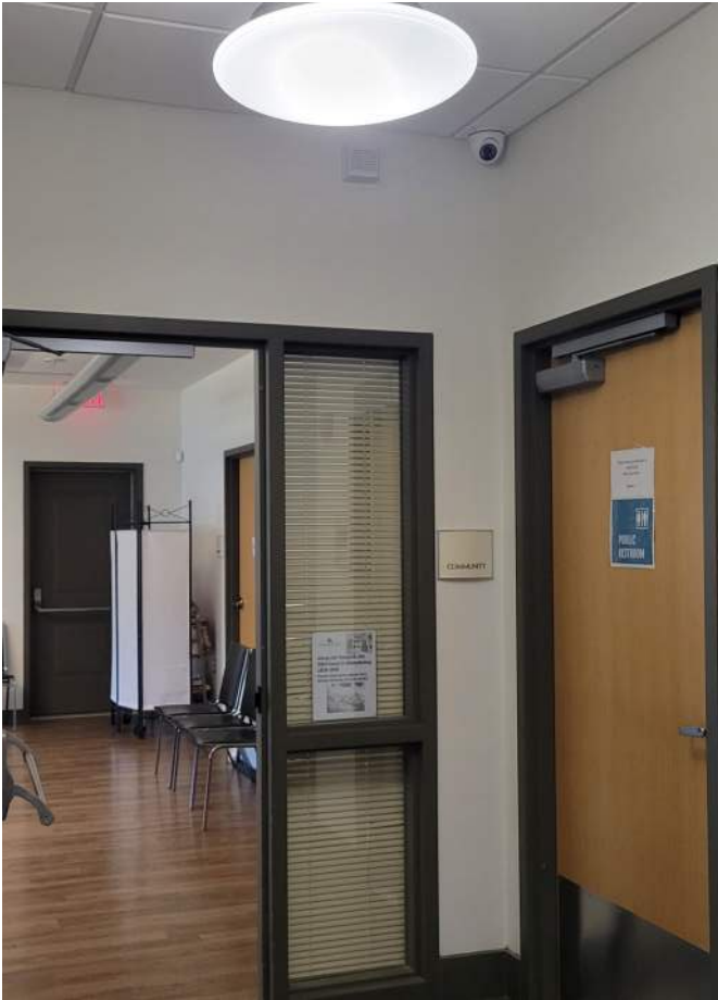
Camera 6 of 8 to be replaced Hallway near bathrooms/entrance
